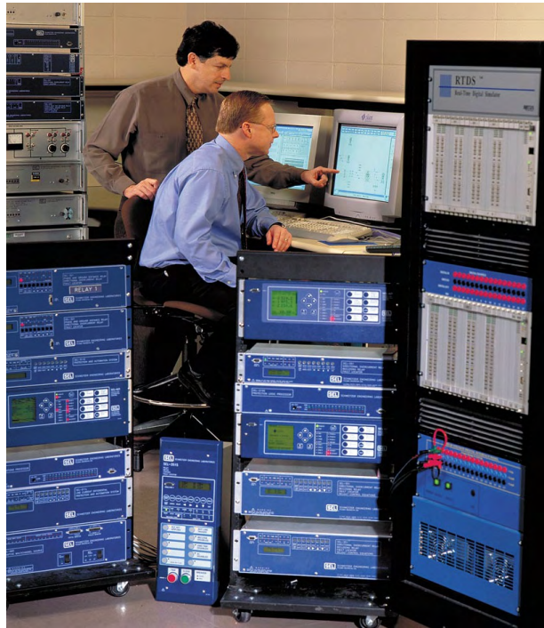
Figure 3 System testing on an RTDS, one of the six owned by SEL
