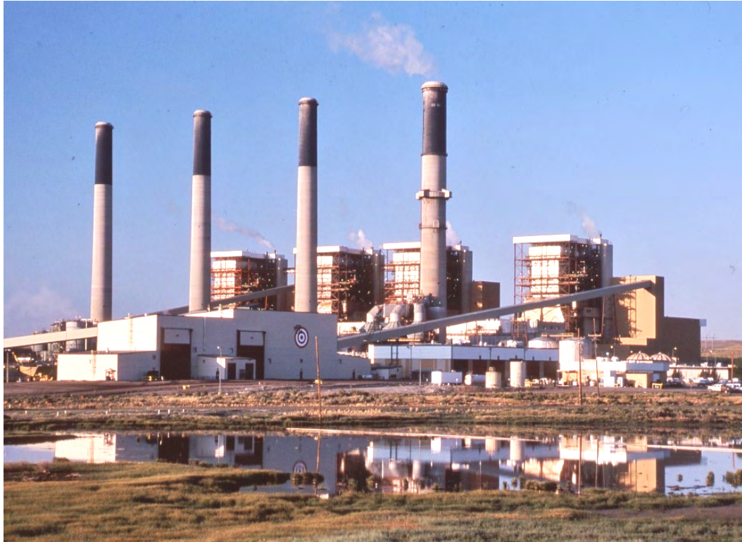
Figure 1 Jim Bridger Power Plant has the fastest triple-redundant system in the world, improving output by 50 percent
