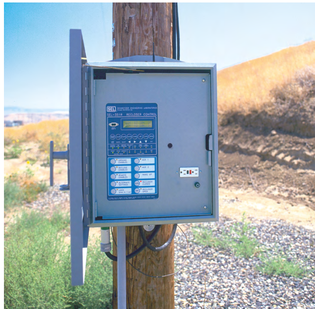
Figure 2 Recloser with Control can be Used for Small Wind Turbine Connection to the Grid
