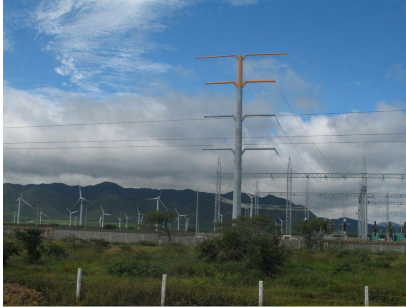
Figure 1 La Venta II Substation Complete Protection and Control Using IEC 61850 Protocol
