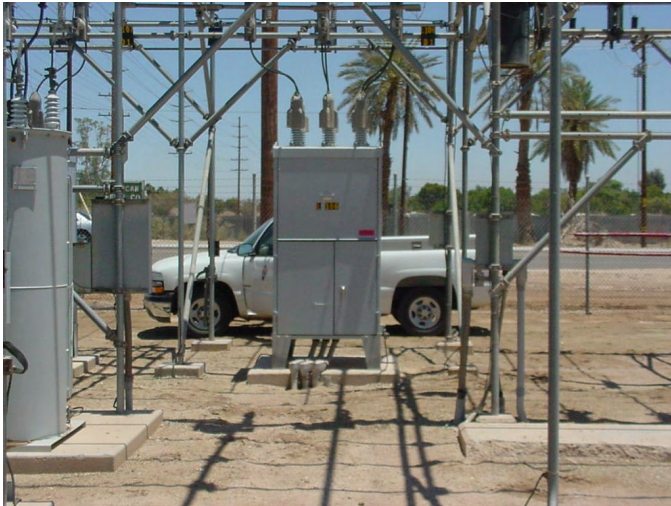
Fig. 1. Euclid Substation in Imperial Irrigation District
