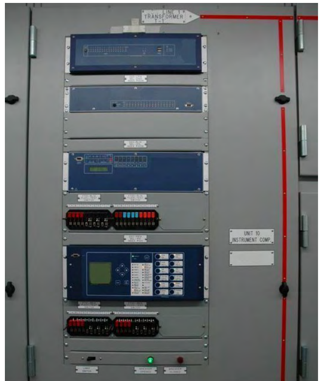
Fig. 12 Switchgear Control Compartment Door
