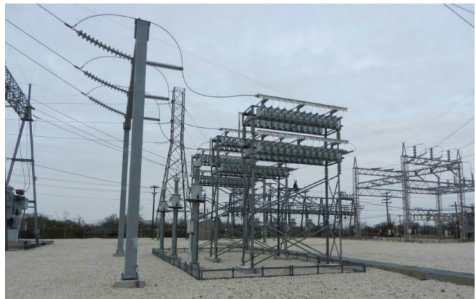
Fig. 1. 31.2 MVAR shunt capacitor bank at 138 kV substation.
