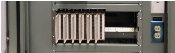
Fig. 4. Transmission line protection panel with installed test blocks at the bottom.
